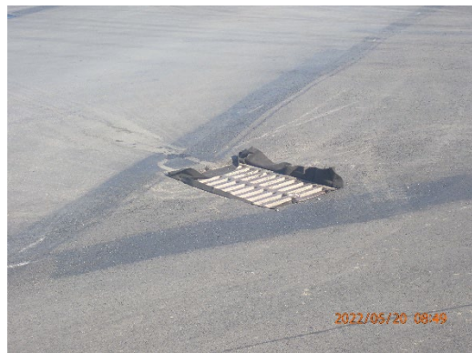
Witches Hat in Storm Water Grate
