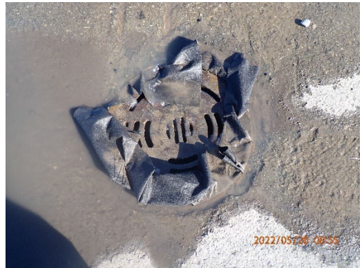
Witches Hat in Storm Water Grate
