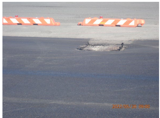
Witches Hat in Storm Water Grate
