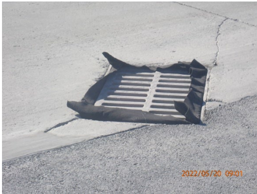
Witches Hat in Storm Water Grate
